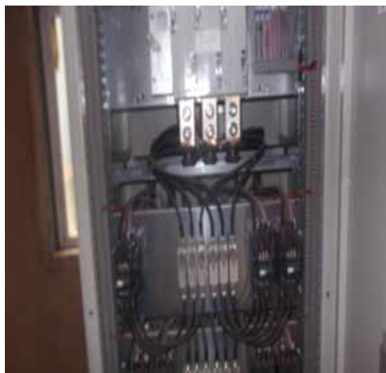
Capacitor banks installed to increase machine efficiency and reduce electricity consumption and hence associated energy consumption cost
