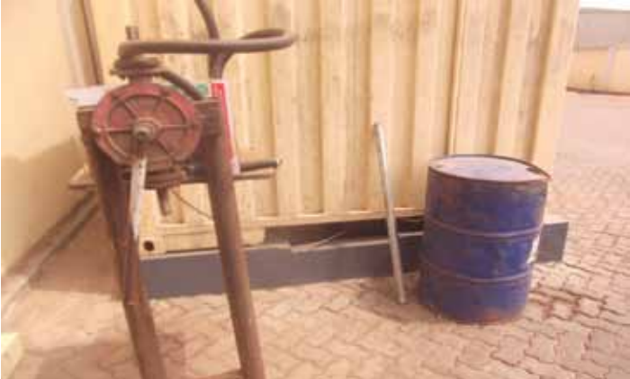
Use of Siphon pumps (in place of manual mode of fetching chemicals etc.) to reduce chemical spillage
