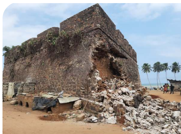
A crumbling wall on the fort at British Komenda. ©UNESCO/George Koranteng
