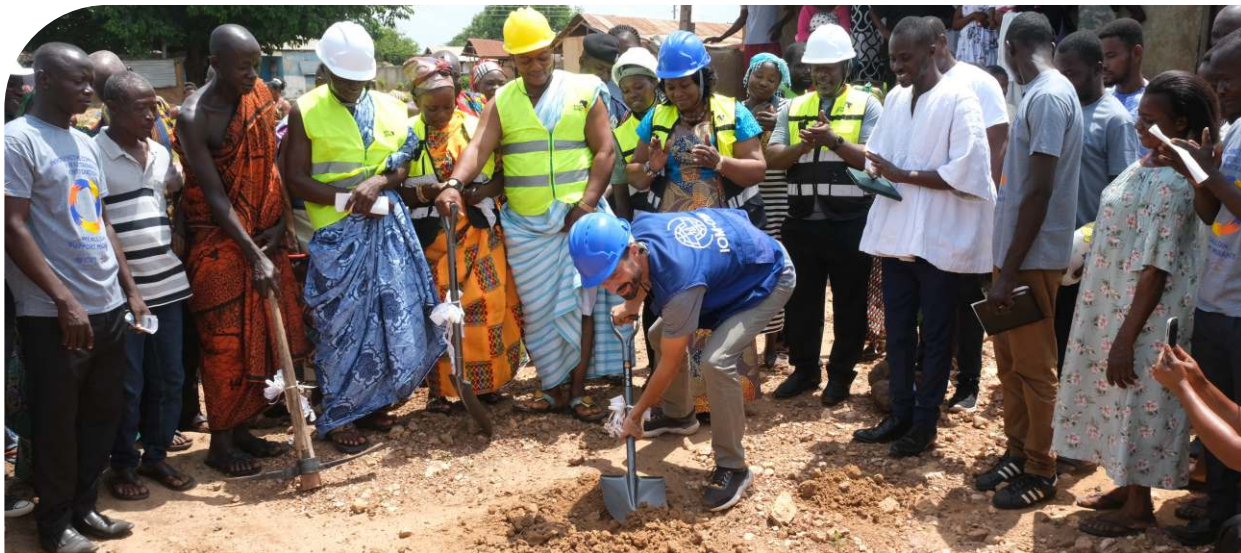
Breaking the ground for a cassava processing factory in Adamu. ©IOM Ghana 2022
